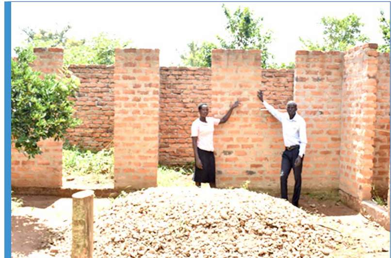
Isaac Toga and his wife stand in front of a brooder house under construction.
