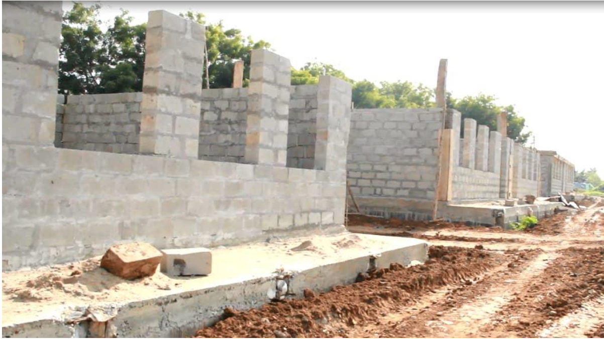
Part of the new school infrastructure for the SEED secondary school under construction in Wadelai Sub county
