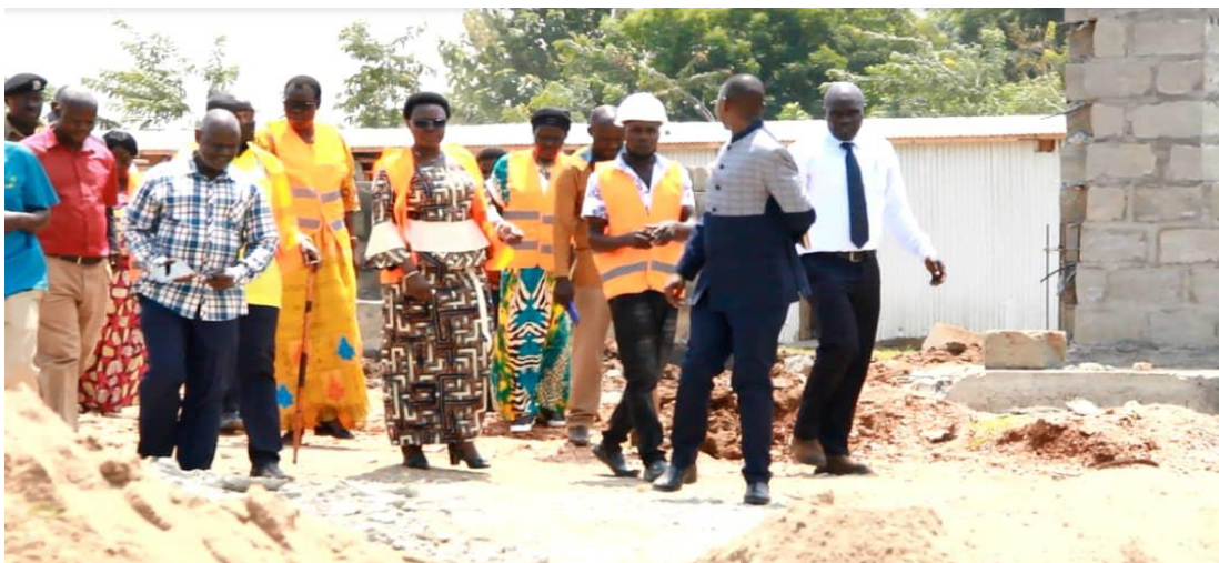
The Hon Minister (middle), Woman MP Pakwach District, The RDC Pakwach and other Stakeholders, on a site visit to Wadelai Seed Secondary School (Under Construction)
